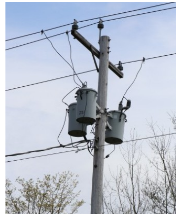
Figure 10.23 A cluster of three residential power transformers.
