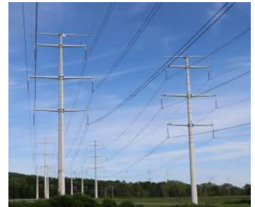
Figure 1.1 345,000 volt transmission lines.
